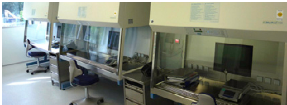
Cleanroom laboratory for cytostatics. CleanSteriCell® GMP A in B with safety workbenches.
