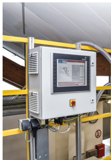
The dosing system is controlled by a Gravinet GP control unit, which is operated using a menu displayed on a 12.1 (Picture: Motan-Colortronic)
