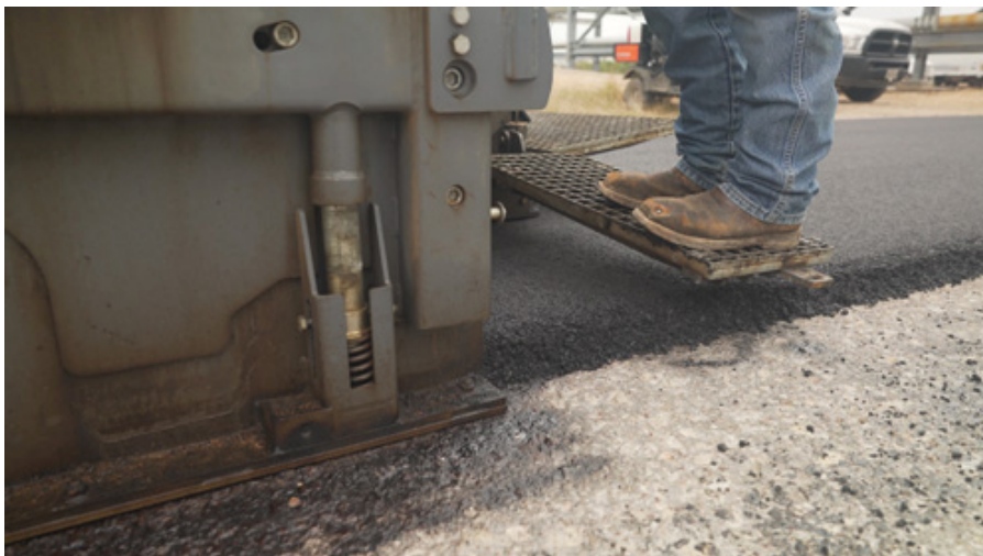
Dow paved two roads at its Texas plant in February with a special asphalt modifier that included LLDPE scrap. The process could become a major recycling option for consumer waste. (Credit: Dow)
