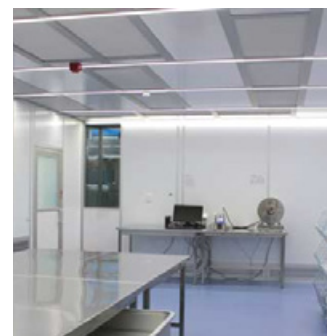
Cleanroom system CleanCell4.0® of the ISO cleanroom class 5. The dimmable LED lighting ensures balanced light in the area of the spreading table.
