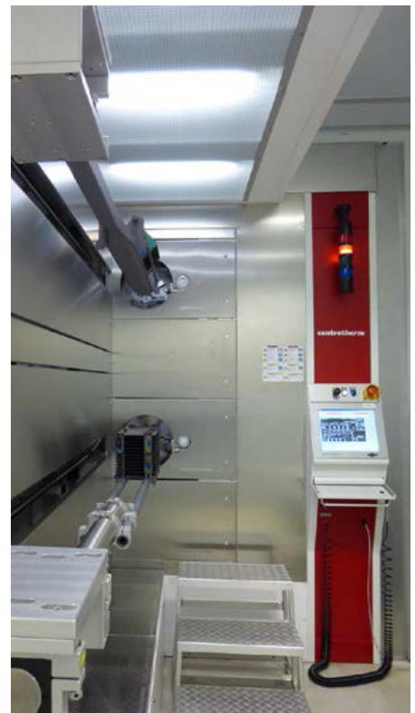
For the cleanroom of Fraunhofer ISE, the consortium implemented a remote monitoring for cells in diffusion tube.
