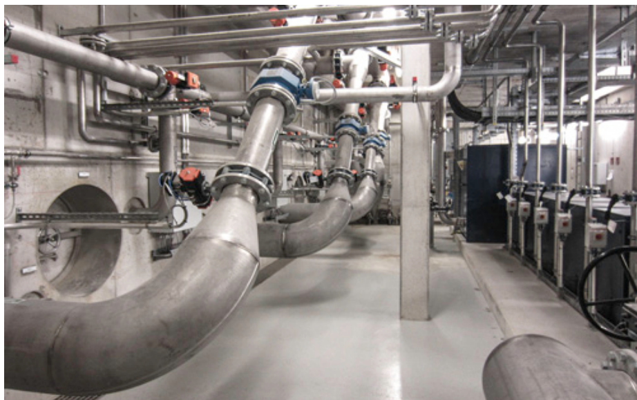
Inlet and Distribution to BIOFIT®.F
