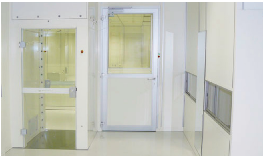
Personnel showers of the personnel airlock into the cleanroom. On the right, the exit and escape door.
