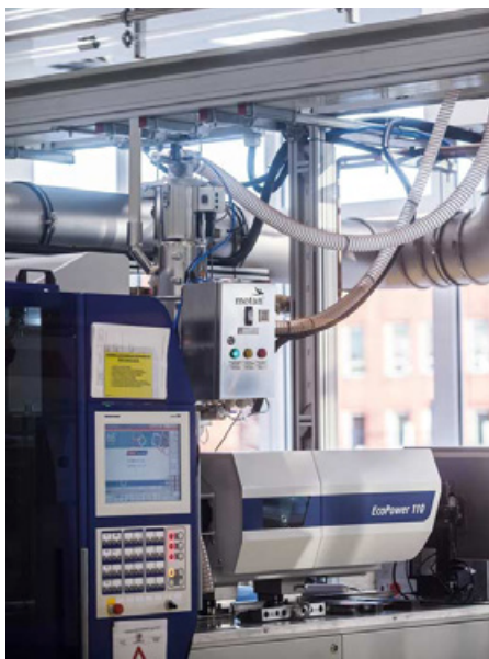
Every compressed air dryer has its own control unit, which communicates with the centralized control system through the Profibus. (Photo: motan-colortronic)
