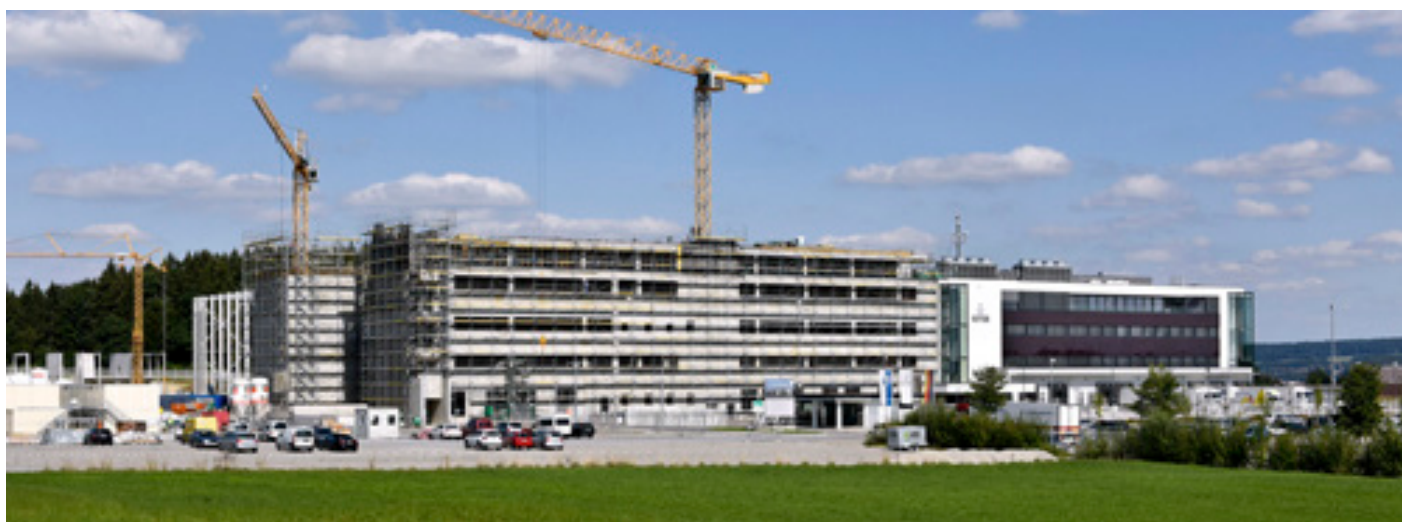
Structural work completed: A portion of the 300 million Euro investment is directed to completion of the Ravensburg Vetter West facility expansion.
